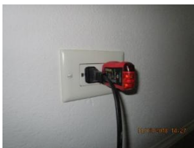
4.16 Receptacle outlet north (N) appeared generally sound.
