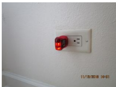
4.81 Receptacle outlet (N) appeared generally sound.
