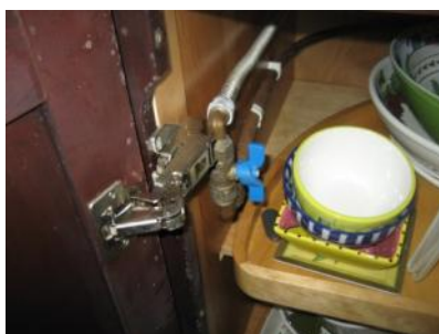
Shut off for gas was located in the cabinet to the right of the stove.
