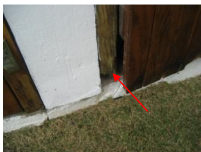
Deteriorated wood frame for the pump room.
