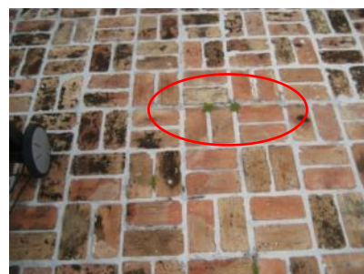
Vegetation growing in the deck should be removed.
