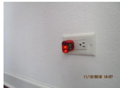
4.14 Receptacle outlet south (S) appeared generally sound.
