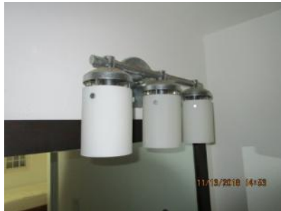
4.87 Fixture appeared generally sound.
