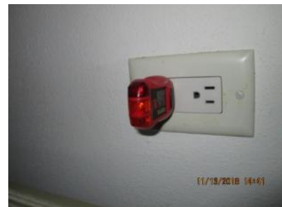
4.53 Receptacle outlet (N) displays a reversed polarity (HOT/NEU); needs correcting.
