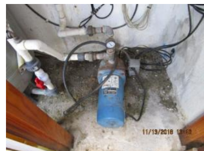
5.1 Pump/Utility Room/ Water Heaters
