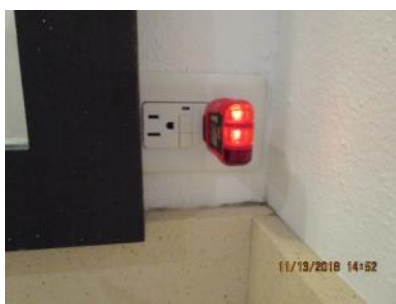
4.85 Vanity GFCI receptacle outlet tested ok; appeared generally sound.
