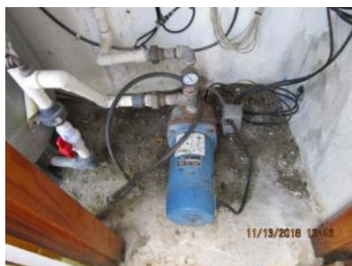
5.2 A domestic water pump located within an exterior utility room near main entry appeared generally sound.
