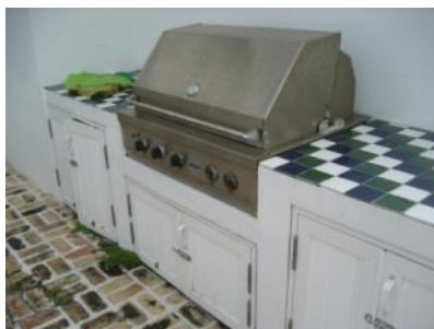
Barbeque on the west porch was not tested. A couple of controls knobs were missing.
