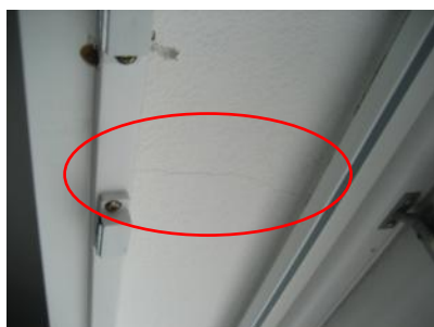
Minor hairline crack was observed in the lintel over the French doors.
