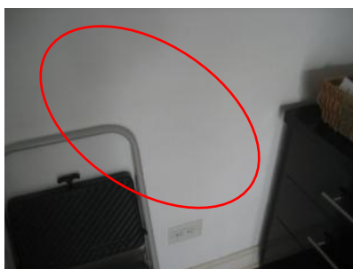
Minor hairline cracks were observed on the west wall of the bedroom.
