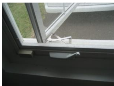
Awning windows operated correctly when tested.
