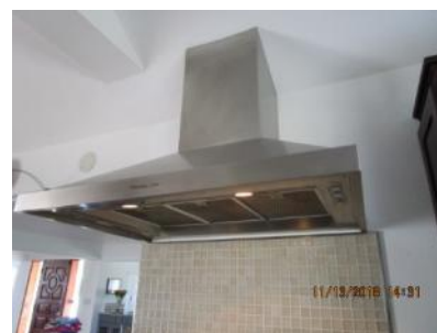
4.32 Exhaust hood tested ok; appeared generally sound.
