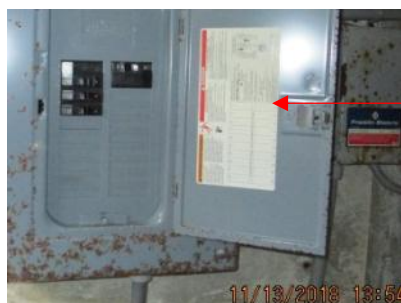
3.6 Panel directory needs to be completed.
