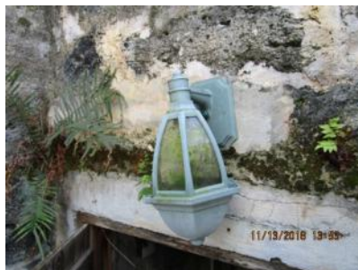
4.102 Fixture (Pool Equipment room) is beyond salvage and needs replacing.
