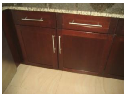
Cabinets were in satisfactory condition,
