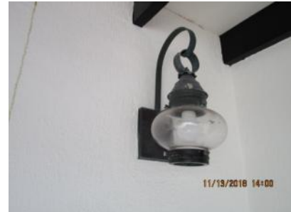
4.107 Fixture (W) appeared generally sound.
