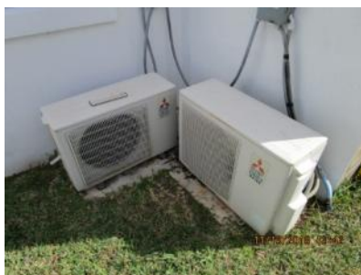
7.2 The Split-Air Condensing units located on the west side of the residence appeared generally sound.
