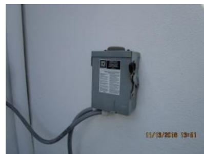
7.6 The disconnects serving the units are per code; appeared generally sound.
