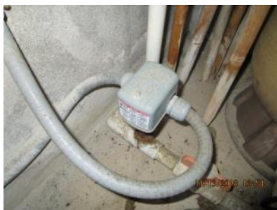
5.6 Pressure switch appeared generally sound.
