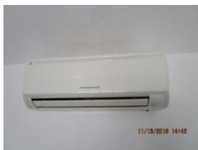
7.13 The split-air-conditioning unit tested ok; appeared generally sound.
