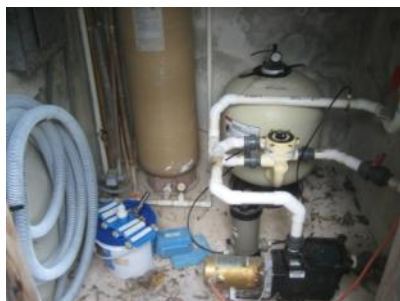
Pool pump room.
