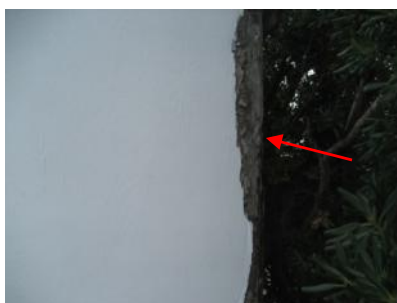
Damage from wood boring insects on the southwest corner of the shed.
