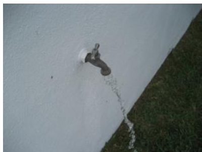
Exterior north faucet tested satisfactorily.
