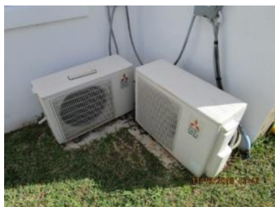
7.1 Air-conditioning/ Swimming Pool
