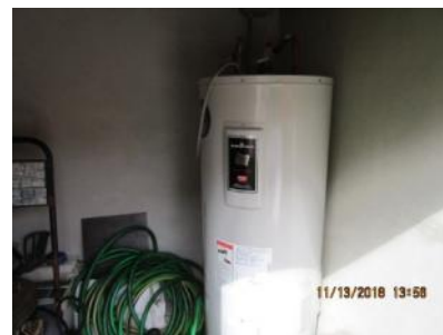
5.7 A domestic water heater located within a utility room south side of the residence appeared generally sound.
