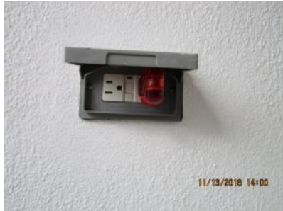
4.105 GFCI receptacle outlet (W) tested ok; appeared generally sound.
