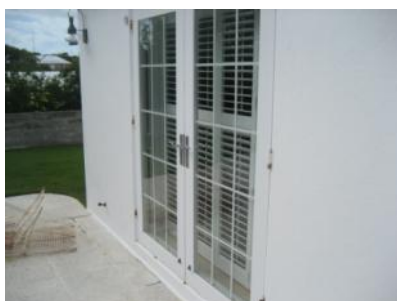
Corroded hinges and hardware were observed on the south French doors.
