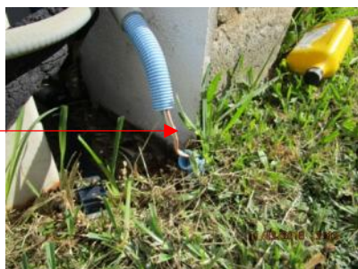
7.4 The E.N.T. conduit (Smurf Pipe) seen here is broken due to physical damage likely from a weed whacker exposing the live conductors. E.N.T. is not permitted by code to be installed in like areas; should be replaced with a more durable type conduit.
