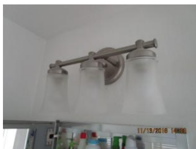
6.63 Fixture appeared generally sound.
