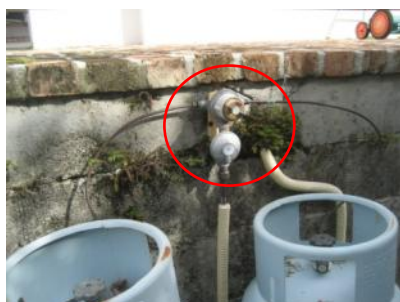
Regulator for LPG tanks.
