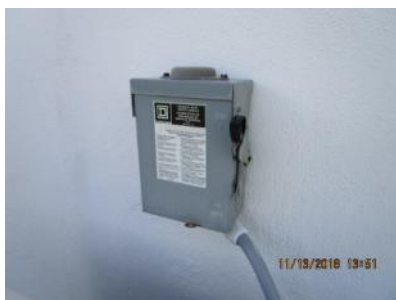
7.8 The disconnect serving the unit is per code; appeared generally sound.
