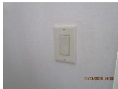
4.23 Switch appeared generally sound.
