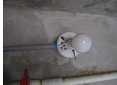
7.21 Fixture appeared generally sound, However, needs a new bulb.
