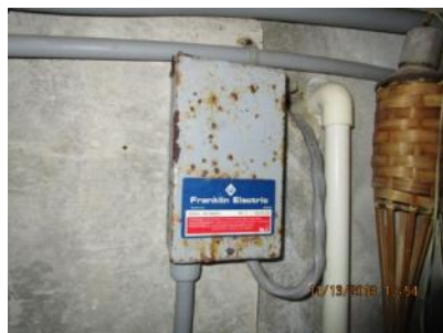
5.5 Well pump controller located in pool equipment room appeared generally sound.
