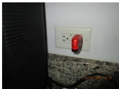
4.27 Counter GFCI receptacle outlet (E) tested ok; appeared generally sound.
