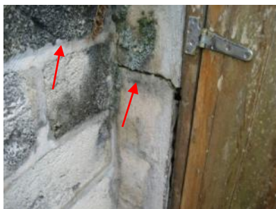
Crack was observed extending into the interior of the pump room along the south wall.
