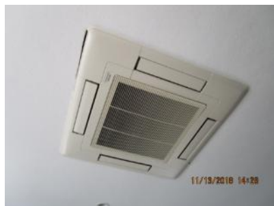
7.10 The cassette split-air-conditioning unit tested ok; appeared generally sound.
