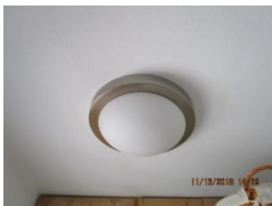
4.22 Fixture appeared generally sound.
