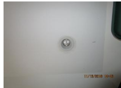
4.59 Exposed bulbs not permitted in clothes closets.
