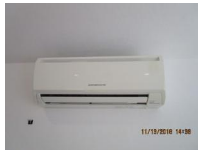
7.12 The split-air-conditioning unit tested ok; appeared generally sound.
