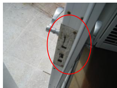
Corroded hardware on the French doors.
