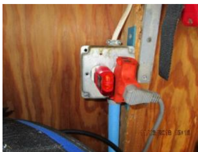
4.109 Receptacle outlet located in shed is required to be GFCI type as per code.
