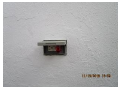
4.104 GFCI receptacle outlet (W) tested ok; appeared generally sound.
