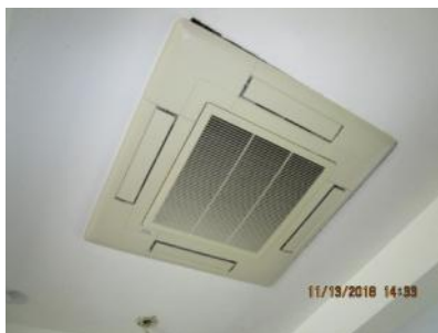
7.11 The cassette split-air-conditioning unit tested ok; appeared generally sound.
