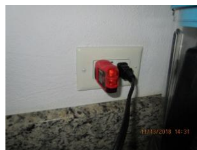
4.26 Counter GFCI receptacle outlet (E) tested ok; appeared generally sound.
