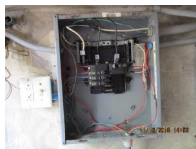
3.5 Circuit conductors and feeders appeared generally sound.
