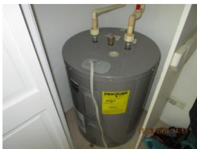
5.12 A 2 nd domestic water heater located within the lower bedroom closet appeared generally sound.
