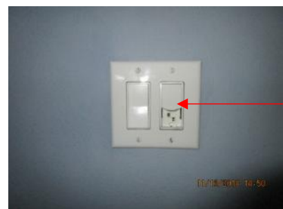
4.77 Combo switch is broken; needs replacing.
