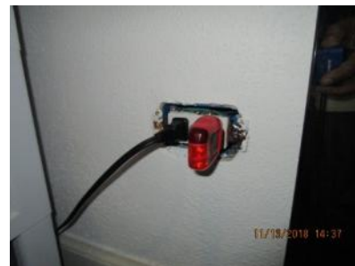
4.44 Receptacle outlet (E) requires a cover plate.
