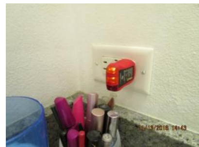
4.62 GFCI receptacle outlet tested ok; appeared generally sound.
