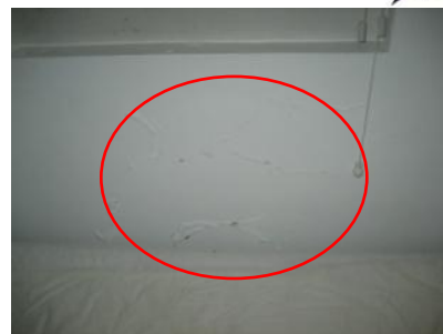
Efflorescence was observed on the south wall of the bedroom.
