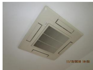
7.9 The cassette split-air-conditioning unit tested ok; appeared generally sound.
