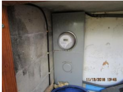
1.1 Service Entrance (Belco Meter) (BTC)
