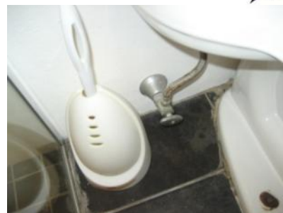
Shut for toilet was present.
