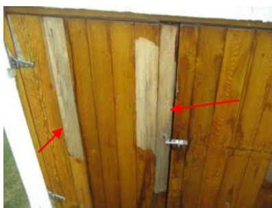
Finish on pump room door was deteriorated. The finish should be restored to protect the wood from deterioration.
