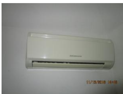
7.14 The split-air-conditioning unit tested ok; appeared generally sound.
