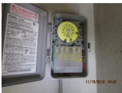
5.9 Time clock is rated for the load; appeared generally sound.
