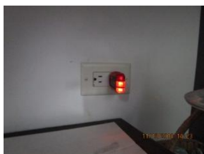
4.3 Receptacle outlet east (E) appeared generally sound.
