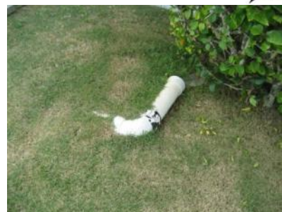
Tank overflow was observed in the north yard.
