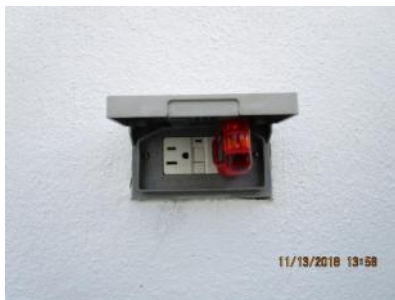
4.103 GFCI receptacle outlet (W) tested ok; appeared generally sound.
