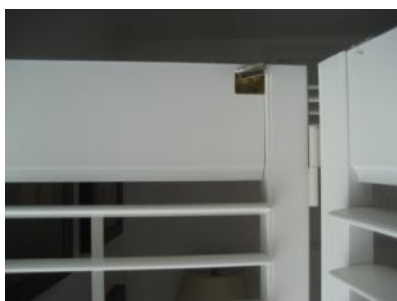
A damaged magnetic latch was observed in the right side of the door.
