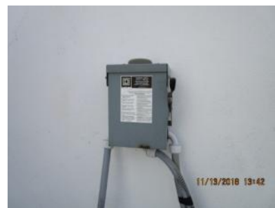
7.3 The disconnects serving the units are per code; appeared generally sound.
