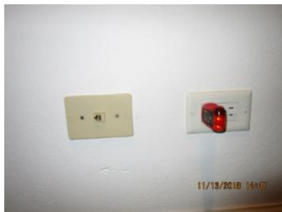
4.69 Data; Receptacle outlet (N) appeared generally sound.
