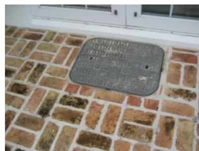
Tank was securely covered and full when inspected.
