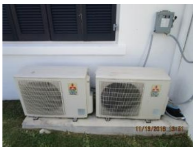
7.5 The Split-Air Condensing units located on the east side of the residence appeared generally sound.
