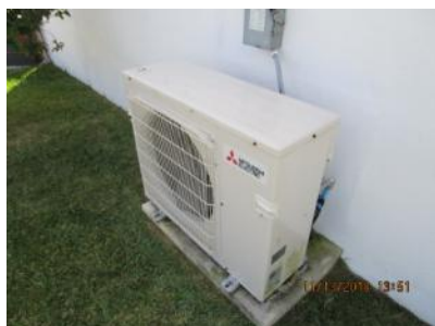
7.7 The Split-Air Condensing unit located on the east side of the residence appeared generally sound.
