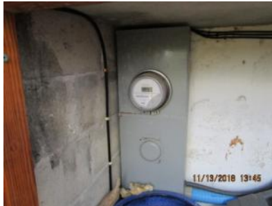
1.2 The residence is supplied with a 200A 120/240V single-phase service located in an exterior utility room west side of the residence. The metered service appeared generally sound.
