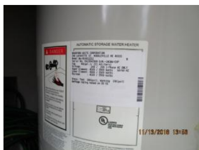
5.8 The water heater has a rating of 4500Watts at 240V for a total of 19A. Circuit conductors are suitable for the load.
