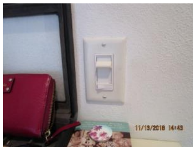
4.60 Switch appeared generally sound.
