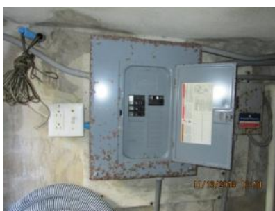
3.4 A 100A 120/240V 06 CCT distribution panel located in the pool equipment room appeared generally sound. However, the panel is starting to rust. Recommend sanding and painting.
