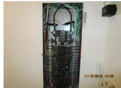
2.2 A 200A 120/240V 32 CCT distribution panel located in the laundry appeared generally sound.
