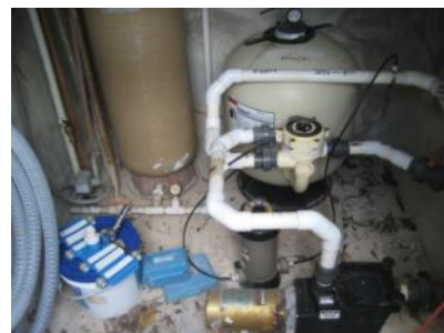
Equipment appeared to be in satisfactory condition.
