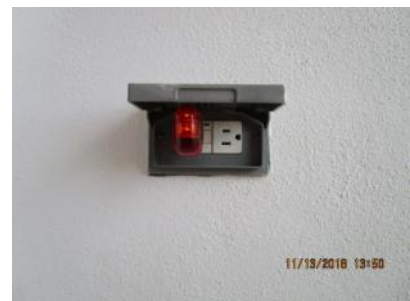
4.95 GFCI receptacle outlet (S) tested ok; appeared generally sound.
