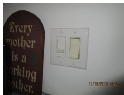
4.5 Switch appeared generally sound. The dimmer however, is faulty.
