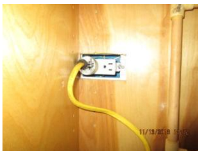
4.28 Under cabinet receptacle requires a cover plate.
