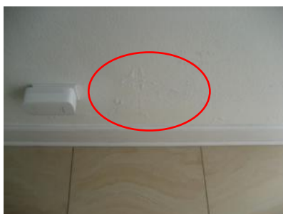
Small amount of efflorescence on the hallway wall.
