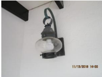
4.106 Fixture (W) appeared generally sound.
